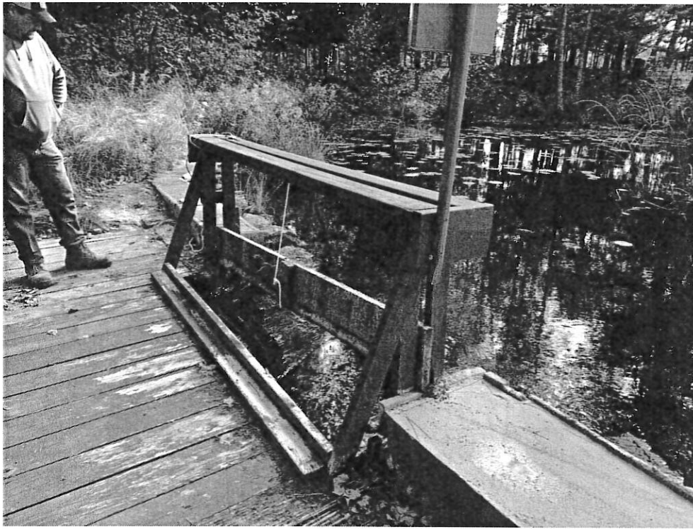
PHOTOGRAPH 5—Stoplog in raised position
